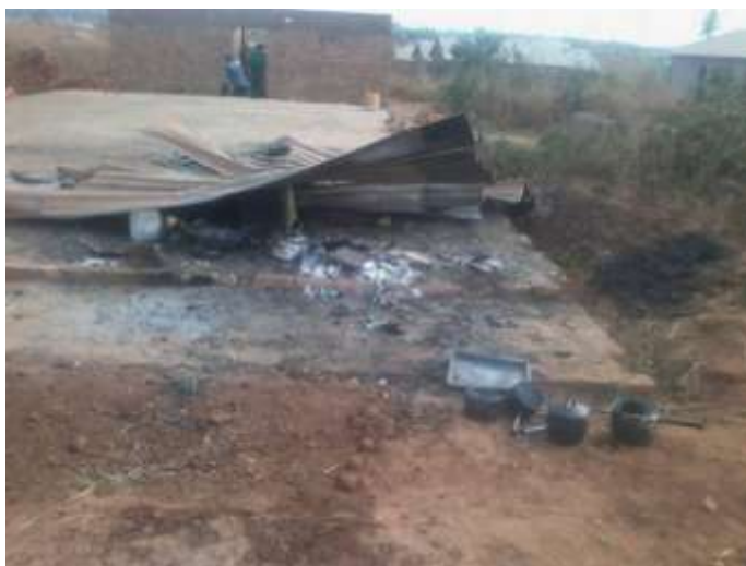
The remains of the structure that was gutted by fire
